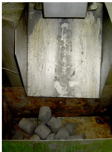
Picture 4: The sludge is automatically pressed into briquets.
