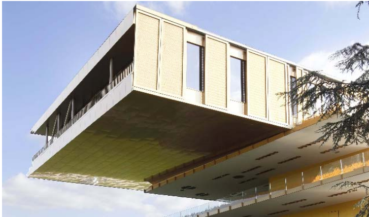
Picture 5: The solar protection panels made of GKD metal fabric of the type ESCALE 7x1.5, which measure more than three meters in height and 1.70 meters in width, protect the building from becoming uncomfortably hot.
