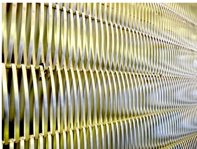
Picture 7: In the foyer of the Tours du Pont des Sèvres Dominique Perrault combines the spiral mesh with its function as discreet screening (Escale 7 x 1) or fall guard protection (Escale 7 x 2).
