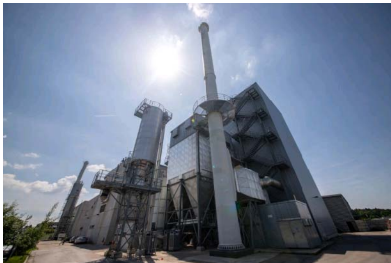
Picture 2: The combined heat and power station with steam turbine has a maximum electrical output of 9.6 megawatts and is fed with 36 tons of steam per hour.
